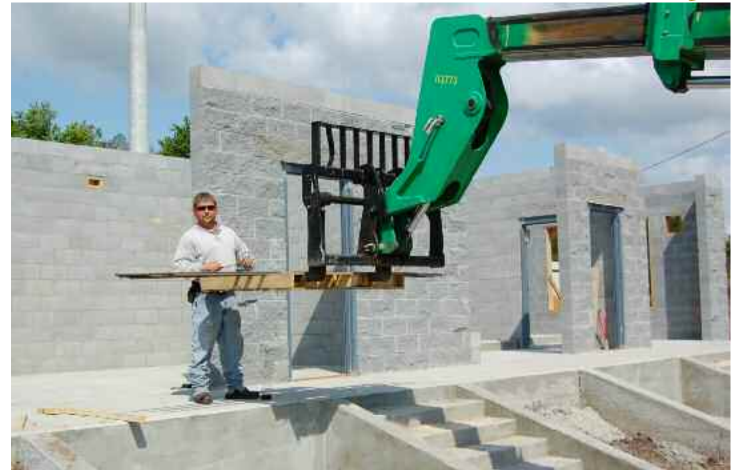
Stacey Hutchinson of HUTCHCO Industrial Services constructs the electrical vault as part of the totally new electrical system at Brunswick Golden Isles Airport.
